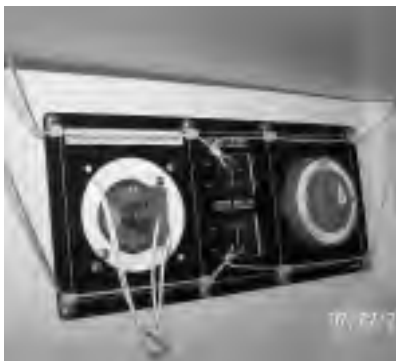
Battery panel with emergency jump to starter switch
