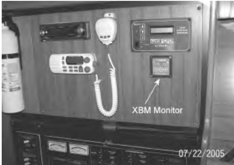
XBM Monitor located above DC panel
