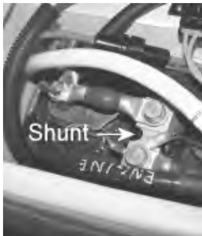
XBM monitor shunt installed
