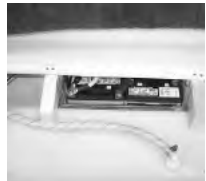
Two PWC batteries next to port side water tank
